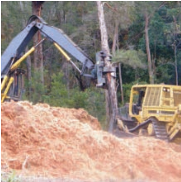
FIGURE 4.4: Tree removal using a claw extension to gently lower trees rather than dropping them. This machinery is suitable when removing habitat trees as it may reduce the impact on any fauna present inside the hollows (Photo: RTA).
