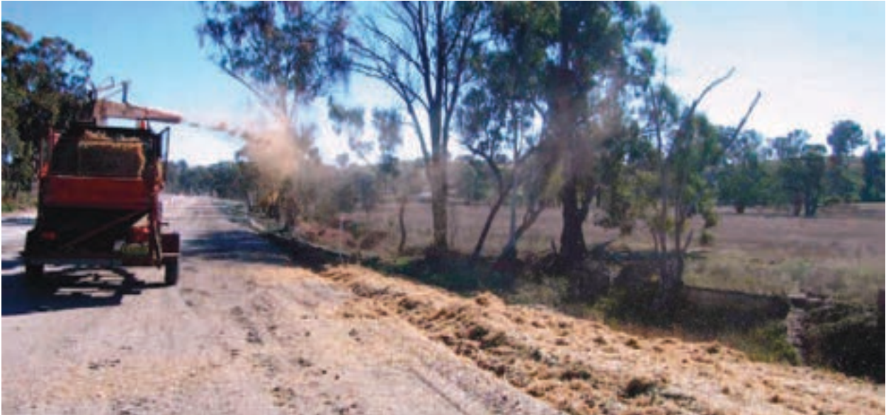
FIGURE 3.8: Strawmulching over a hydroseeded embankment. A tackifier (adhesive) is sprayed over the straw to bind it in place. The materials used must be appropriate to the local context, and consider fire risk, high wind and erosion profiles (Photo: Leigh Trevitt).
