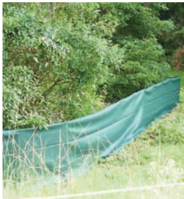
FIGURE 9.8: Temporary frog fencing installed for the Sapphire to Woolgoolga project to prevent the endangered Giant Barred Frog ( Mixophyes iteratus ) from entering construction areas (Photo: Josie Stokes).
