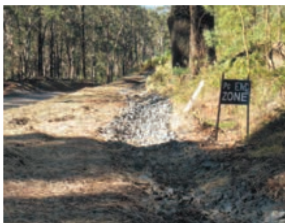
FIGURE 7.10: Pythophthora management measures on the Main Road 92 near Nowra, Southern Region (Photo: Scott Fayers).
