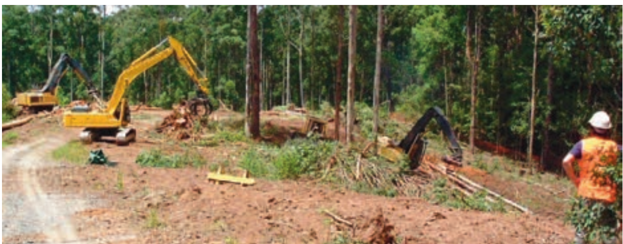
FIGURE 4.1: Staged habitat removal taking place to minimise impacts on biodiversity (Photo: RTA).
