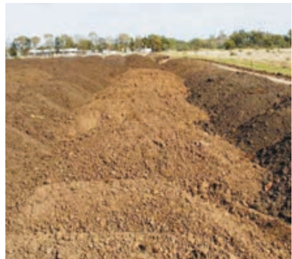
FIGURE 3.3: Topsoil being stockpiled at Moree for re-use later in revegetation and landscaping works (Photo: Lester Piggott).
