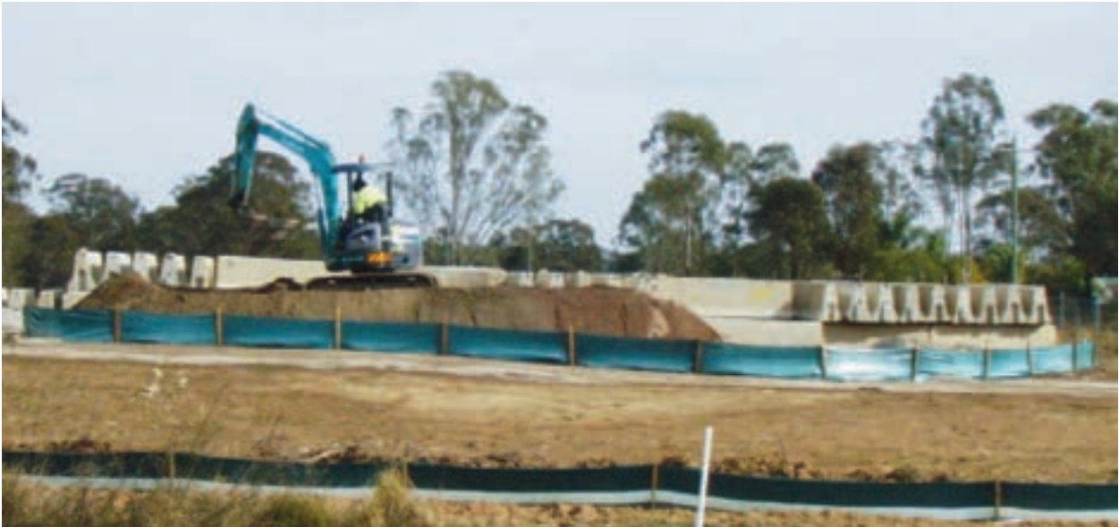
FIGURE 2.9: An example of good practice. This stockpile has been established away from the tree dripline and has appropriate erosion and sediment controls in place (Photo: Dylan Chresby).
